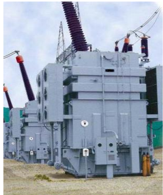
TPP Šoštanj, Slovenia (2005) Installation of on-line monitoring system on two step-up transformers
